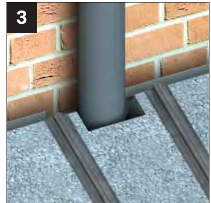
3 The "pipe" panel is cut on site to accommodate the pipe passing through the roof, and the OSB also requires an aperture cut (see inset image).
