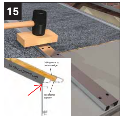
When aligned (ensure external panel clip butts upto aluminium gutter channel, see red arrow) use a robust mallet to knock down the external panel locking clips (use a short length of timber to protect the clip from indentations).
