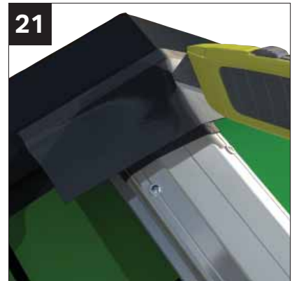
21 Fit second 200mm Butyl tape sealing the dry verge to the gable flashing. Cut the tape to allow it to be folded as shown in the following two images
