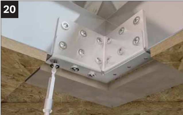
20 The screws to the underside not accessible when box beam sat on brickwork or super insulated columns.
