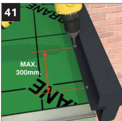
Fix the dry verge to the roof deck with NTRS 050 screws, max 300mm centres.
