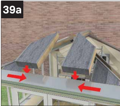
Next, install Ultrapanel working from each hip bar towards the centre Do not cut the binding cords.
