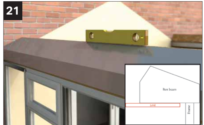
21 Check all is level - pack off top of frames if necessary. CHECK THE UNDERSIDE OF THE BOX BEAM IS LEVEL PRIOR TO FINAL FIXING. PROP IF NECESSARY.
