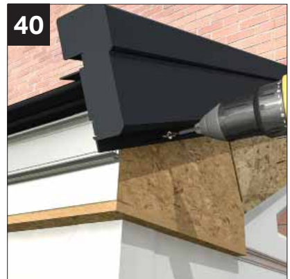
Fix the dry verge to the OSB using NRTS 050 screws at 300mm centres. Ensure membrane overlaps into dry verge for drainage.
