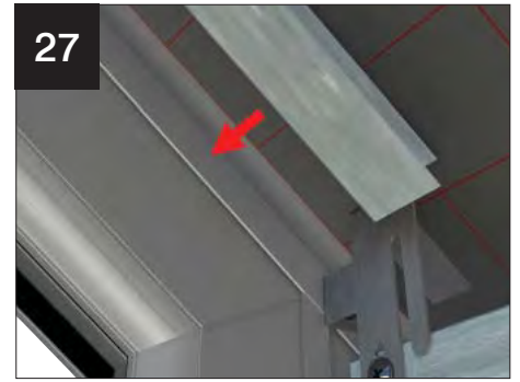
27 Now fit living room channel to gable- this is used to carry 25mm insulation and to secure timber battens and plasterboard adjacent to the gable.
