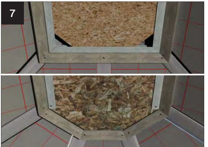
This is how battens should look round Georgian end (top) and Victorian end (bottom).
