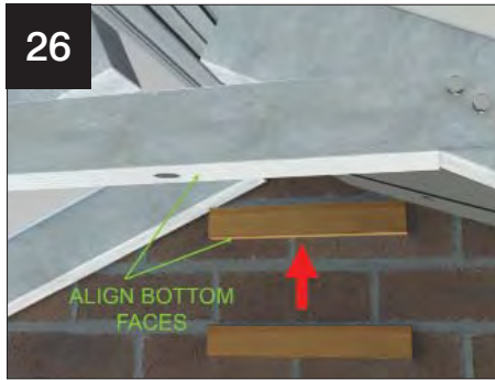
Fit a length of timber batten to the host wall, ensuring that its underside lines through with the underside of the struts (LVTS001/LVTS002). This will provide a fixing point for the ridge board fitted in the next step.
